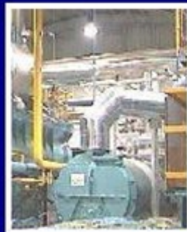
↑ Energy Utilisation Heat Exchanger / Steam Boiler.
