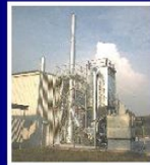
↑ Air Quality Control System.
